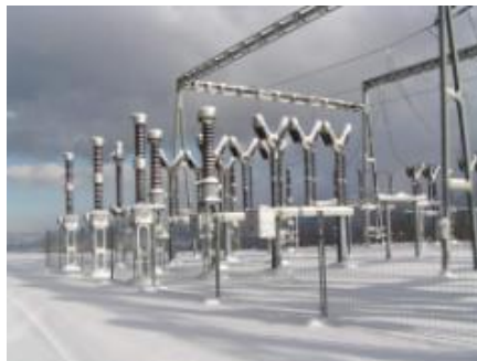
220 kV Switchyard Chavalon Power Station - Switzerland
