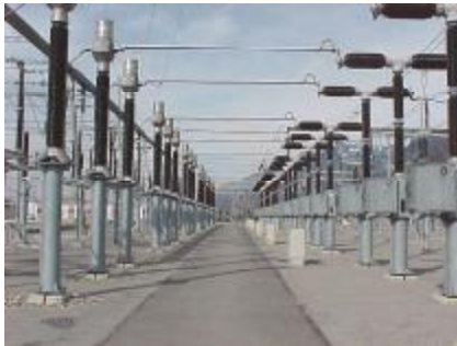
220 kV St-Triphon substation Switzerland
