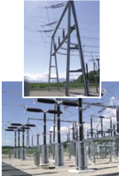
220 kV substation of Crans-Céligny, Switzerland
