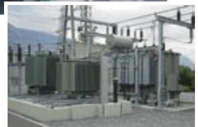
65 kV substation of St Triphon, Switzerland
