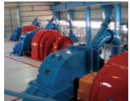
Commissioning of the 3 x 5 MW Sahaniivotry Power Plant, Madagascar
