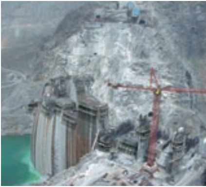
Shahryar (ex Ostour) Arch Dam, Iran
