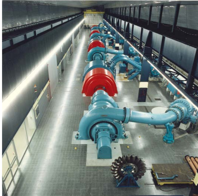
Figure 2: Machine room in Veytaux plant (4 groups of pump/turbine)
