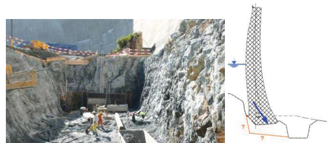
Figure 3: Rehabilitation of Les Toules arch dam, Bloc 6, Excavation of the local deepening of the strengthening
