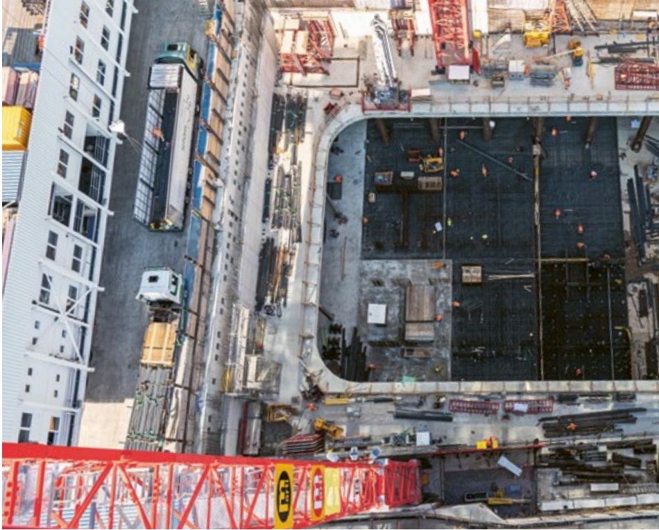
Although Building 2 will be taller than Building 1, various optimizations achieved time and cost savings on the foundations.
