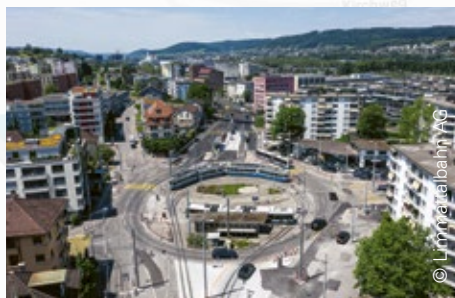
The turning loop for tram line 2 had to be removed within six days ...
