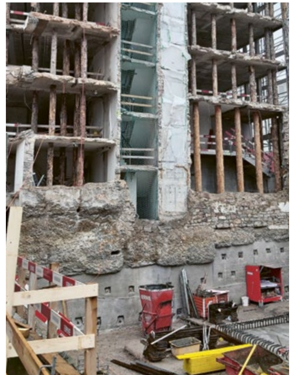
Timber logs were used as props for the stripping and demolition works to the corner building.
