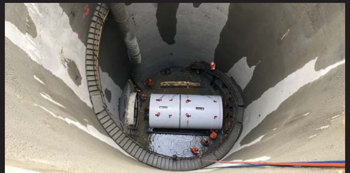
Lausanne Train station, Installation of the Tunnelling Boring Machine for the creation of Cable Gallery under the station, Switzerland
