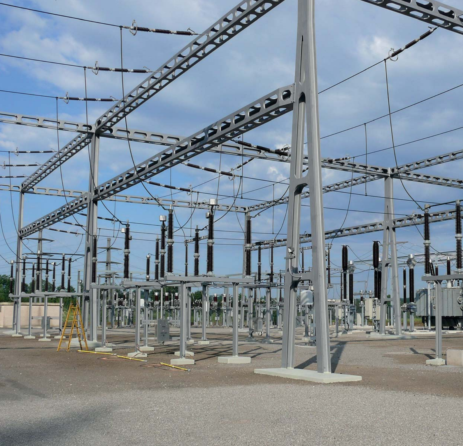
Substation Hauterive, Switzerland
