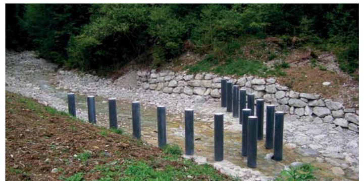
Debris Rake on the Marivue River, Switzerland
