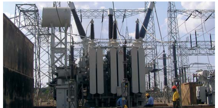
NIPP Transmission lines and substations 330-132 kV, Nigeria
