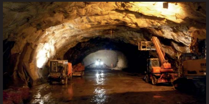
Powerhouse Cavern, Hongrin-Léman Pumped Storage Scheme, Switzerland
