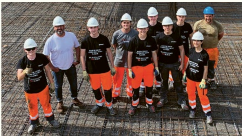
Tired, but happy faces: the trainees are making progress in erecting the new dairy cow barn.
