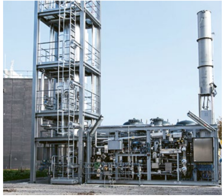
Aarmatt hybrid plant, Solothurn, allows sector coupling of the gas, district heating and electricity networks
